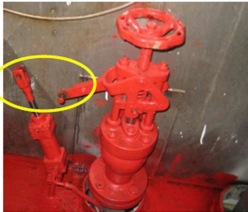
Disconnected control cylinder
