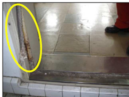
Detached fire door packing
